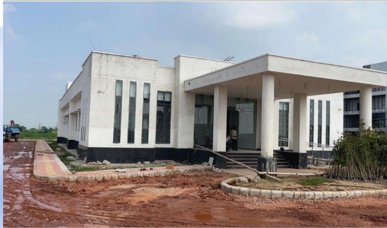
3-D view and actual view of CSF-1: Common IT Facilities
