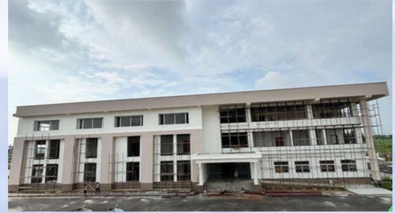
3-D view and actual view of CSF-3: Electronic System & Design Facilities
